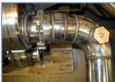
Figure 16 Smoke Port on Inlet Pipe
